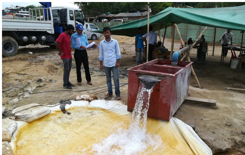
Pump testing of IOM, JICA, DPHE joint water supply project in Camp 12.
