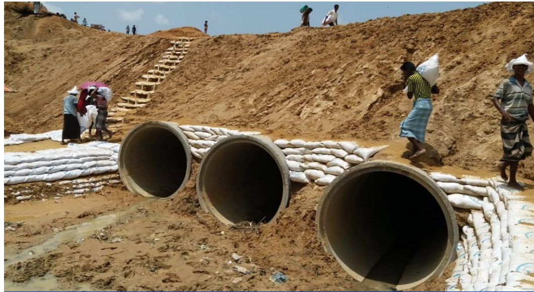
Culverts are being constructed in ten different locations on Army Road in preparation for the monsoon season. All the pipes have now been completed. ©IOM 2018
