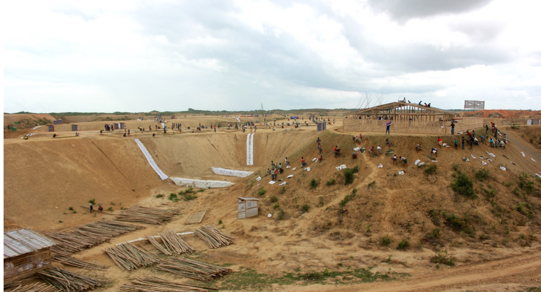
Preparations for the relocation of 1,600 families at risk of landslides and flooding in Camp 20 Extension are ongoing with the construction of the Shelter/NFI distribution point. ©IOM 2018/Mariel Kislig
