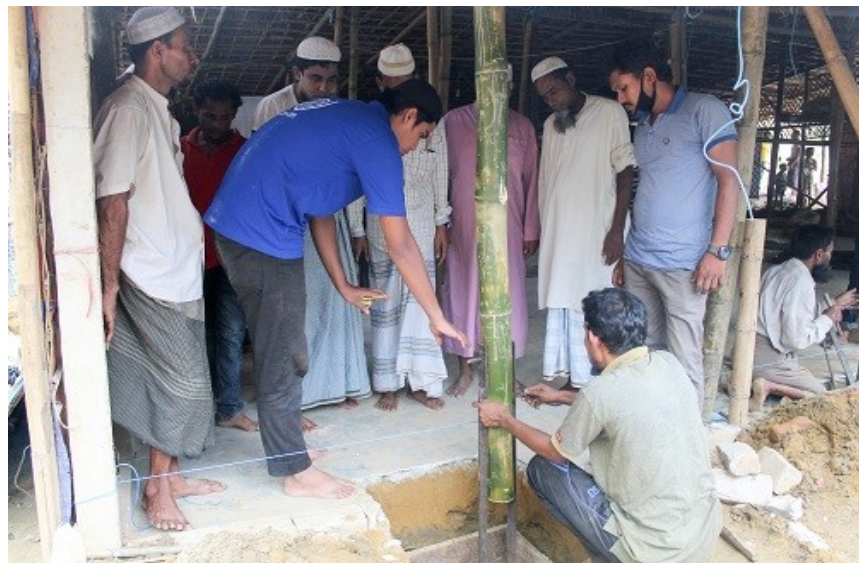
A total of eight mosques are being upgraded with cement concrete foundation, creating temporary communal shelter for 430 individuals in Camp 8E, 9 and 10 of KBE. ©IOM 2018
