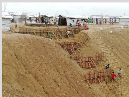
Soil stabilisation by the joint IOM/WFP/UNHCR Site Engineering and Maintenance Project (SMEP).
