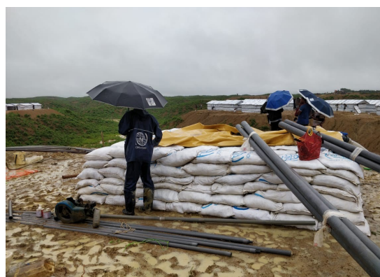
Installation of the second water emergency system in Camp 20 Extension. ©IOM 2018/Rigan Ali Khan
