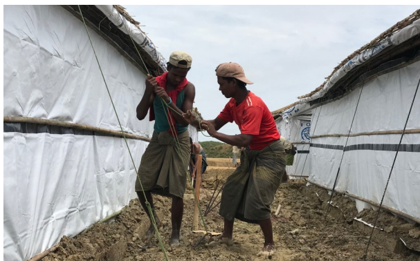
In the mid of the monsoon rains, IOM is prioritizing the application of Tie Down Kits for shelters. ©IOM 2018
