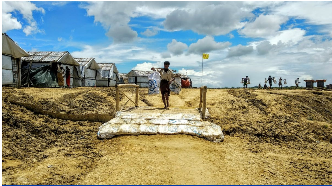
Completed pathway construction in Camp 20 Extension improving access for relocated families. @IOM 2018/Kazi Samrat
