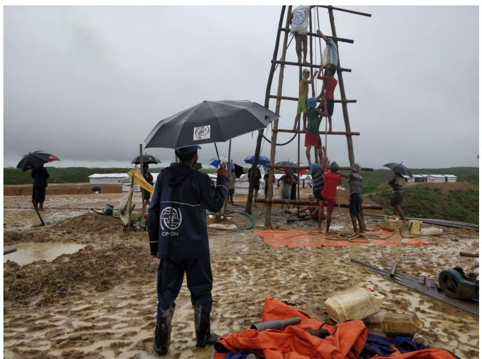
Lowering of Deep Tube Wells (DTWs) ongoing on for new DTWs in Camp 20 Extension. @IOM 2018
