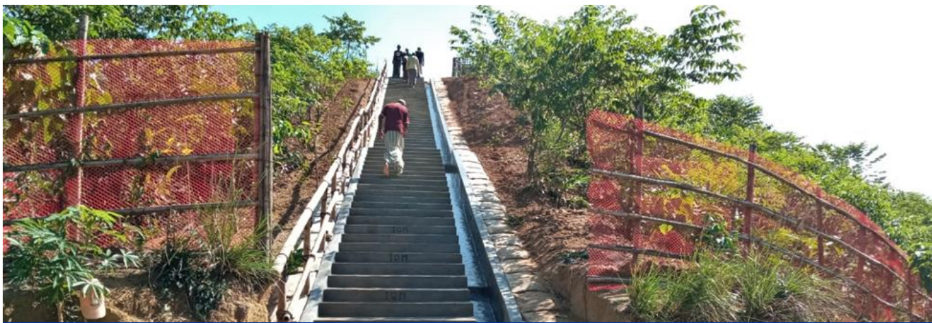
This month, the site development team completed a set of stairs for the graveyard in Camp 20. © IOM 2020
