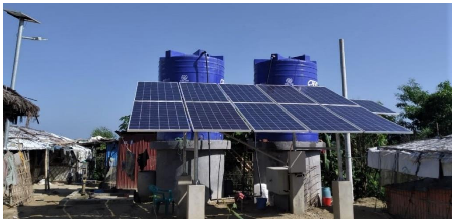
This month, the team installed a small-scale solar water network at Camp 20 Extension. © IOM 2020
