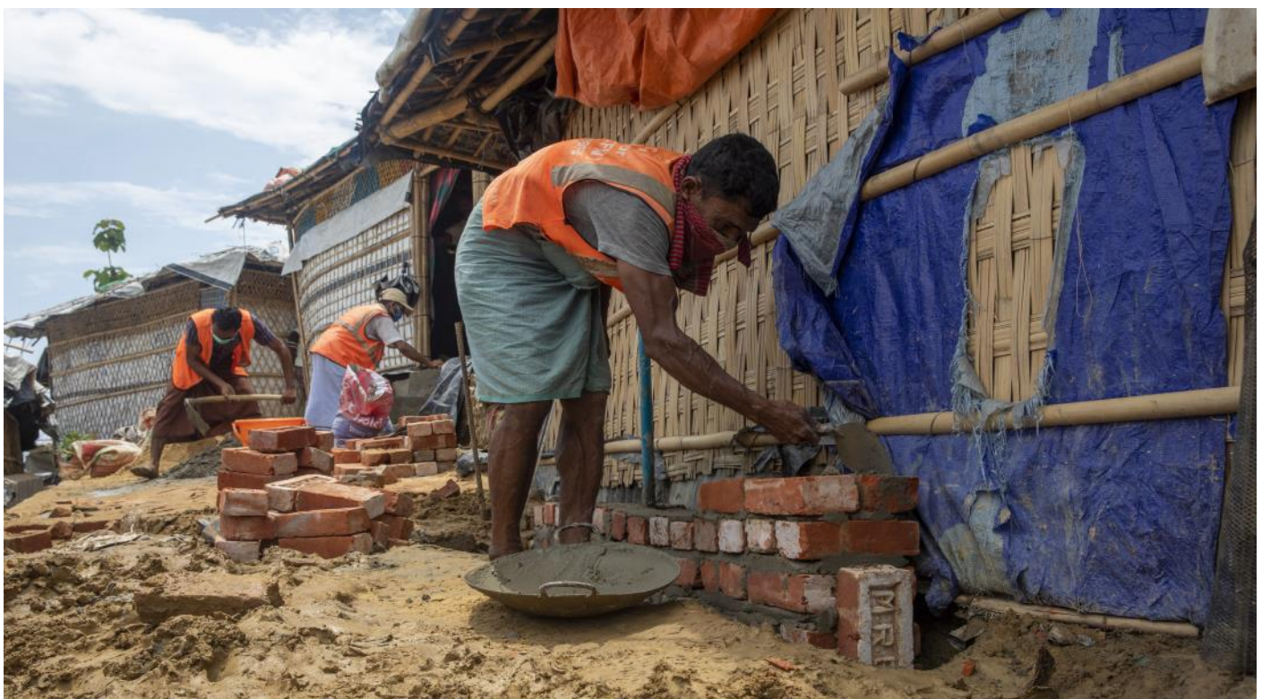
ROHINGYA CASH FOR WORKERS CARRY OUT SIDE PROTECTION WORK ON SHELTERS IN THE KUTULPALONG BALLUKHALI CAMPS © IOM 2020
