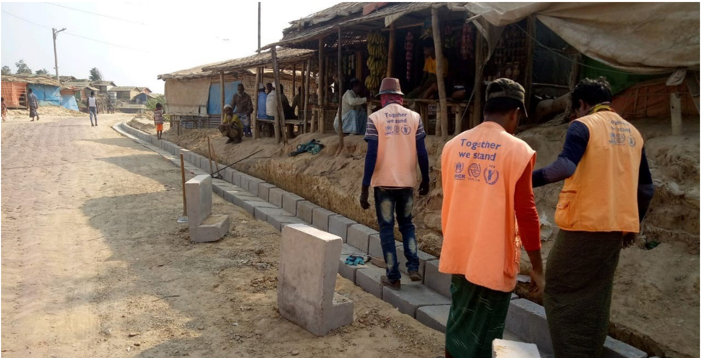
SMEP TEAMS CARRY OUT CURB AND GUTTER INSTALLATION ON ARMY ROAD IN KUTUPALONG-BALUKHALI EXTENSION CAMPS © IOM 2020
