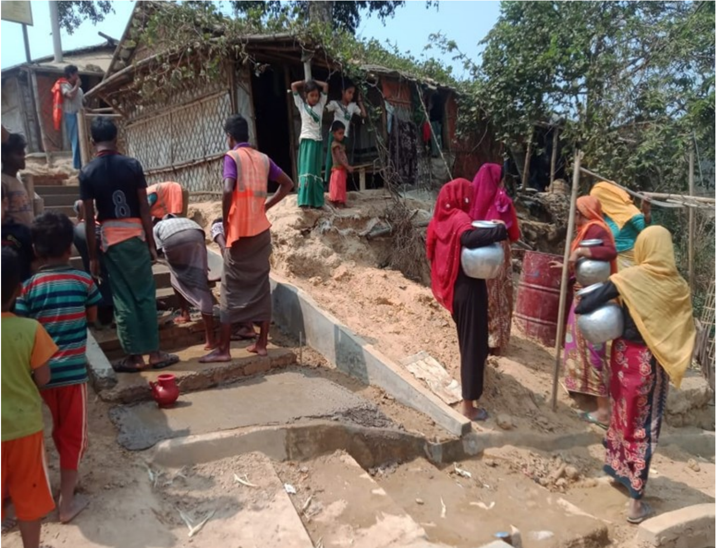
CONSTRUCTION OF STAIRS CARRIED OUT IN EARLY MARCH BEFORE SOCIAL DISTANCING WAS ENACTED — A COMMUNITY WORK FLAGGED BY THE WOMEN'S GROUP IN CAMP 10 © IOM 2020
